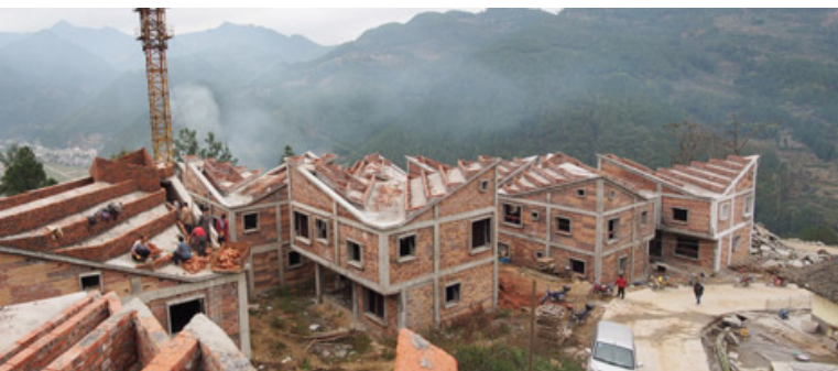
Rural Urban Framework constructed new houses in Jintai Village following the 2008 earthquake and 2011 landslide
